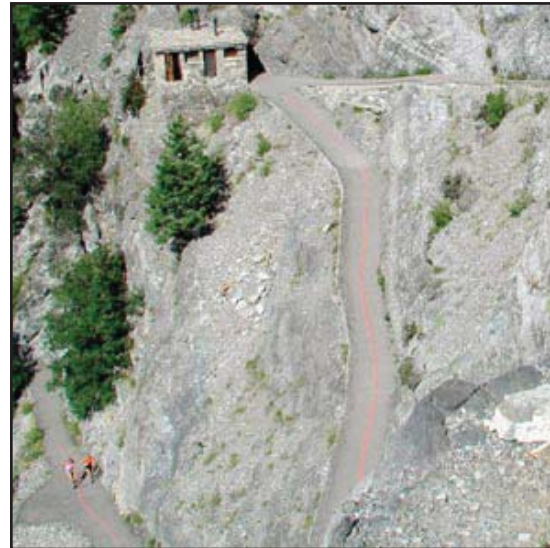
Rockfall danger to the trail as seen from the cave entrance looking northwest. Note the visitors on the trail in the bottom left and the loose rockfall debris directly above and below them. Red lines on trail warn visitors of dangerous rockfall areas. (Photo courtesy of J. Jasper)
