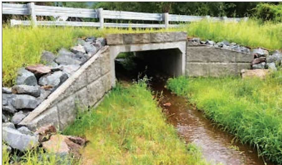
↑ The new culvert on Mill Village Road in Deerfield improves water flow and public safety. (Photo courtesy of Massachusetts EEA)
