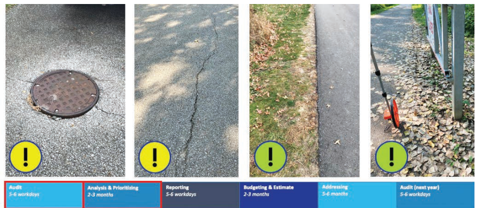
↑ Smaller cracks, bumps, and obstructions are noted and put on the less urgent list. (Screenshot courtesy of the City of Des Moines)
