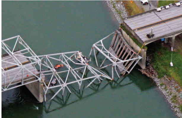
↑ Part of the Skagit River Bridge collapsed when a tall semi-truck, driving in the wrong lane, struck its trusses.
